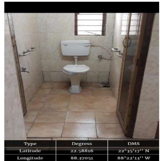
TOILET FOR PHYSICALLY HANDICAPPED
