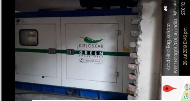
GENERATOR AT PREMISES NO 1
