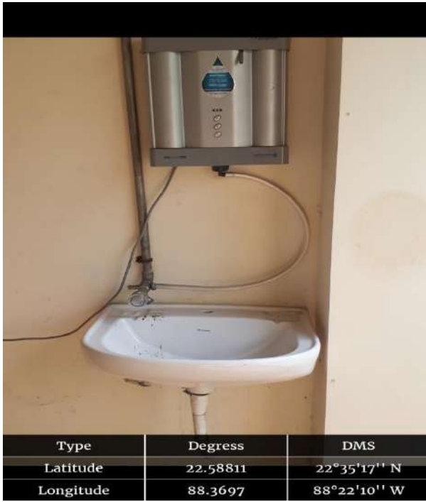
Water purifier at Jubilee Bld (2 nd Fl.)
